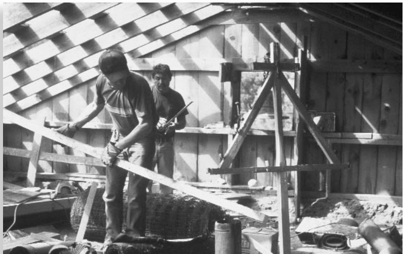
A technical assistance program of Cornerstones Community Partnerships in Santa Fe trains community residents in adobe construction and conservation techniques, to preserve the cultural heritage of New Mexico. Here volunteers make extensive roof repairs to the Nuestra Señora de la Asuncion church in Placita. Photo by Ed Crocker.
